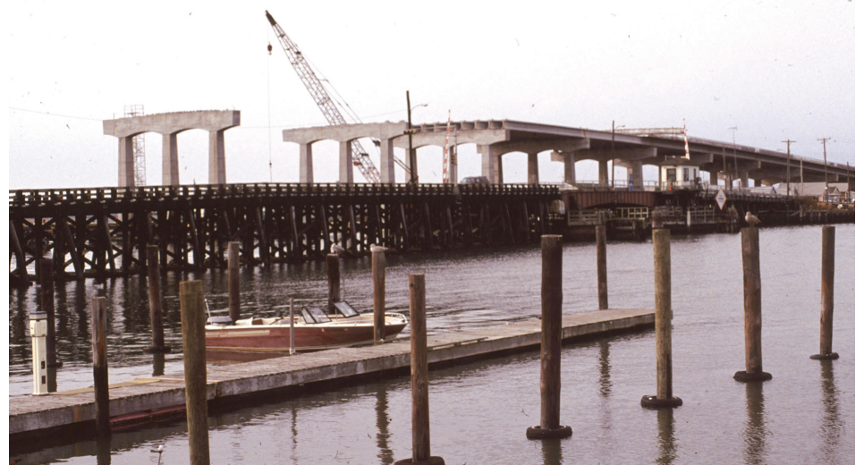
Road and bridge construction on North Wildwood Blvd. began in the late 1980s
